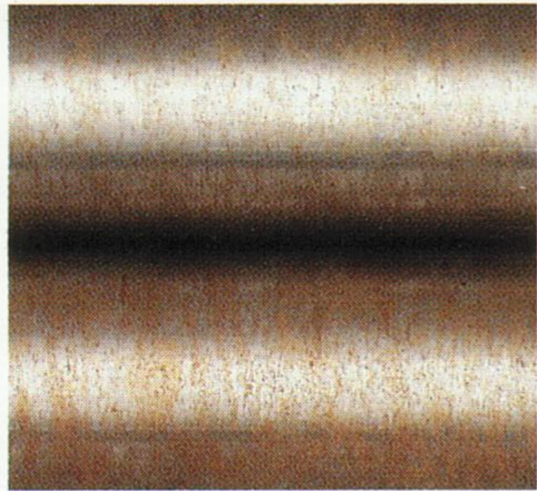
Stainless exposed for 3 weeks to sea spray and groundwater containing sulfides, corrosion so severe that handrails were removed after 3 months.
